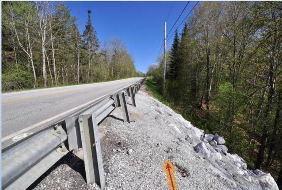
Additional Slope Failure
